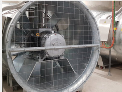
UNDERGROUND L5 ERNEST LLUCH BARCELONA (SPAIN)
