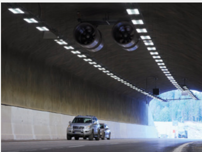
VT1 2 TUNNEL LAHTI (FINLAND)
