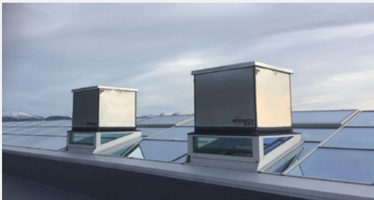
SMOKE EXHAUST Romsdal High School, Norway
