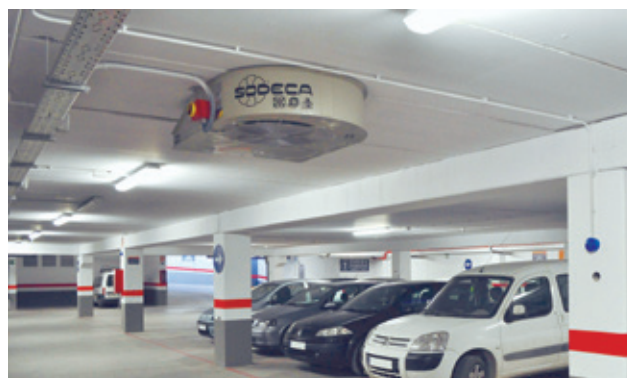
CI installed in car park
